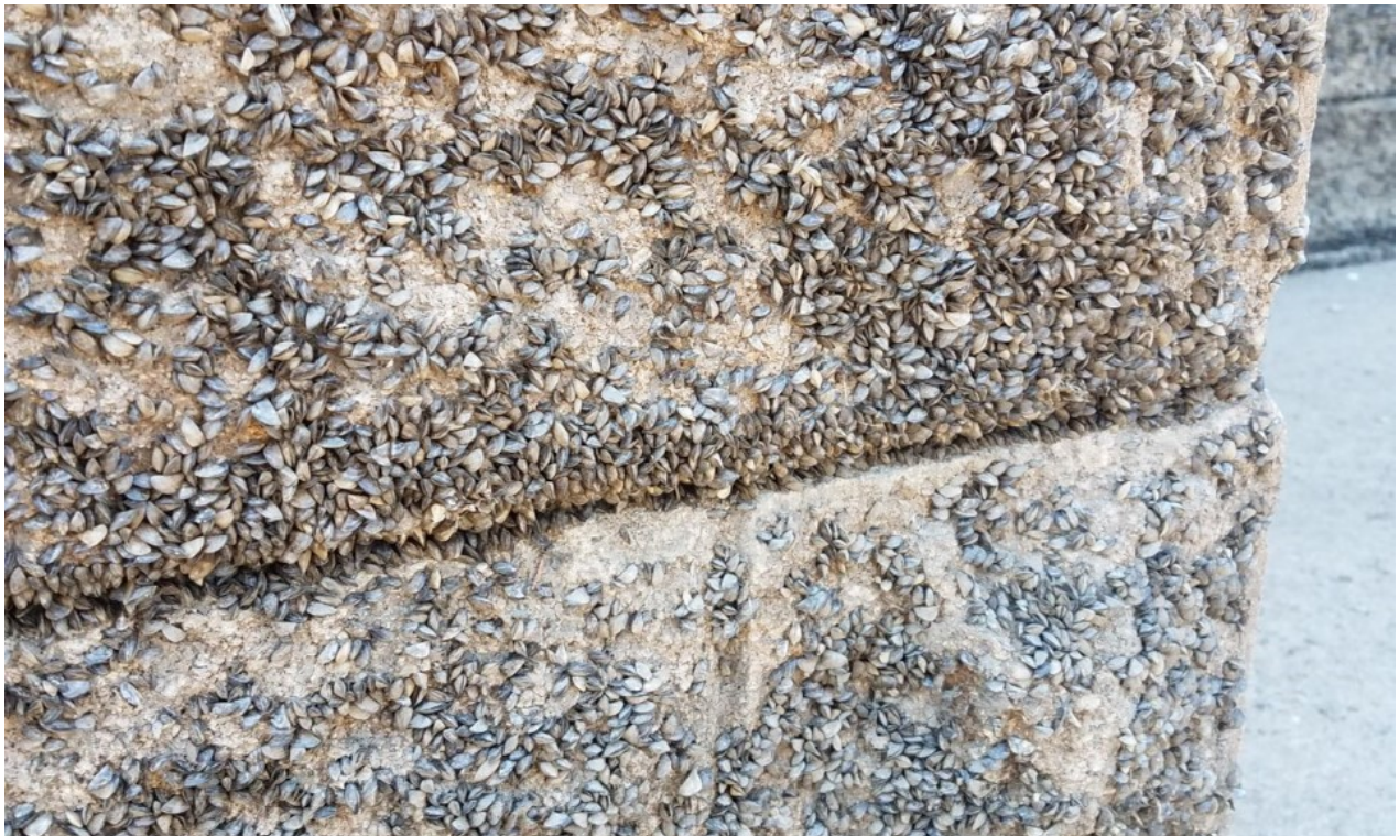
Zebra mussels attached to a State Park shelter that was flooded
