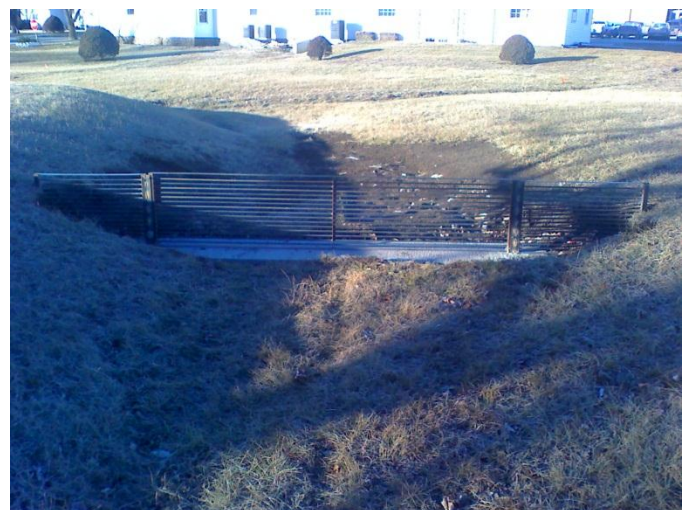
Fish Screen Across Olpe Jones Park Pond Spillway
