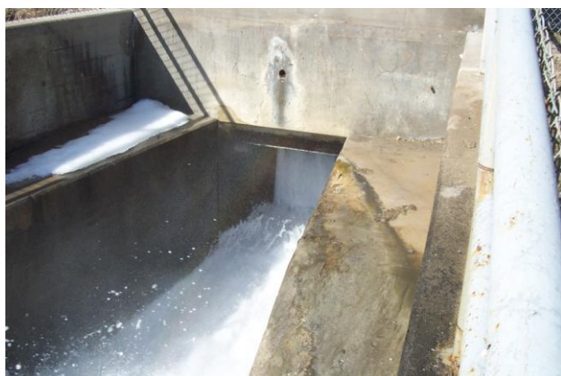
Release water rushing through the gate below the control house
