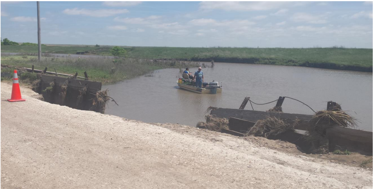
Damage on the road on the west end of HorseThief Reservoir from high water flow.
