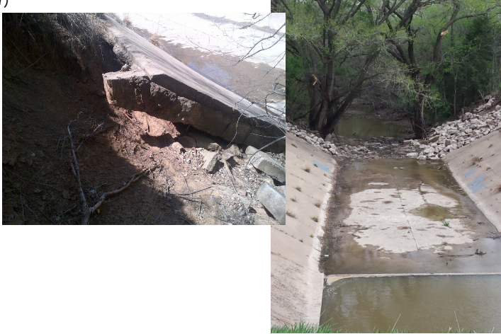
Erosion on the outfall structure on the inlet canal west of the Area office (left) and the rip-rap placed to repair it.
