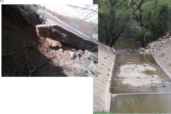
Erosion on the outfall structure on the inlet canal west of the Area office (left) and the rip-rap placed to repair it.
