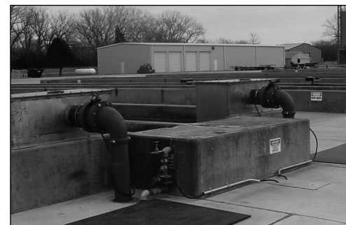
RW Aeration Chamber
