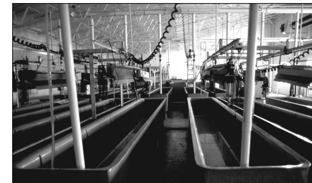
Start Tank Room
