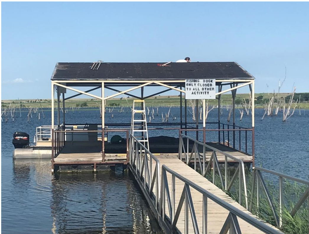
Cedar Bluff fishing dock during roof tear-off, note the habitat barge on the far side of the dock used to contain and transport torn off shingles and tar paper back to the shore for disposal
